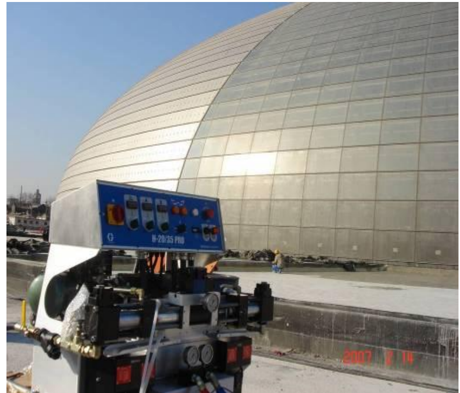
National theater water pool protection
